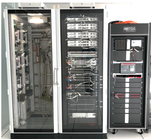
The RTDS Simulator connected to the PMS in RTE International's lab
