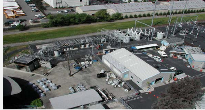
High Current Yard (HCY) T&D equipment testing up to 90,000 A (9,000A at distribution voltage)
