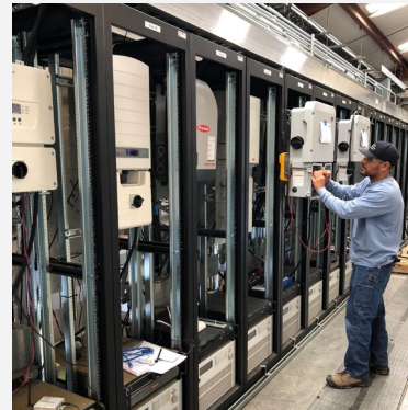
Modular Generation Test Facility (MGTF) DER testing up to 500 kVA
