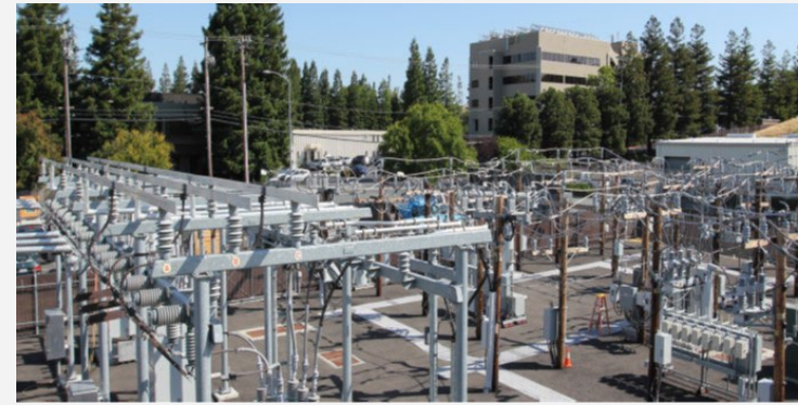
Distribution Test Yard (DTY) Distribution hardware and automation testing
