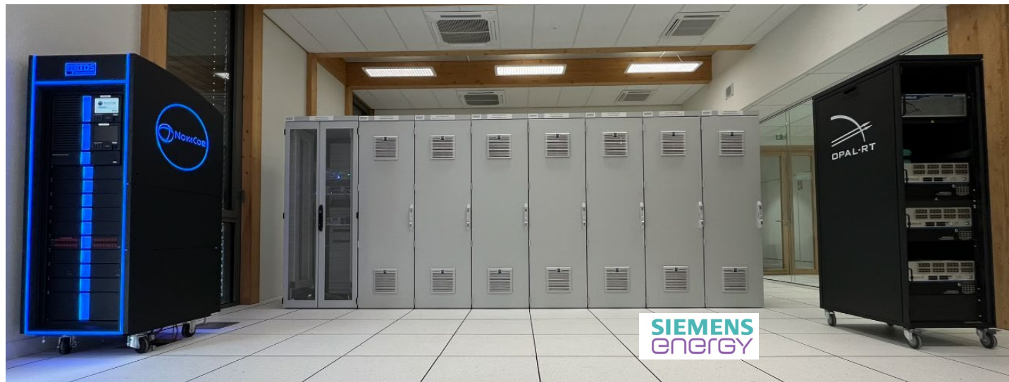
SIEMENS Energy C&P replica installed in RTE lab in July 2024 for InterOPERA project
