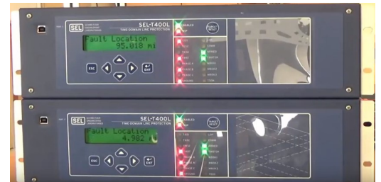
SEL's new T400L (Time Domain Protection) connected in the loop with TWRT
