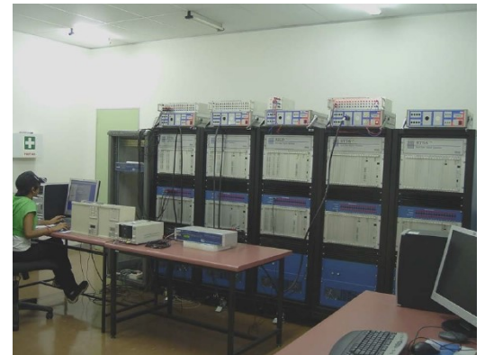
The Real Time Power System Studies Centre
