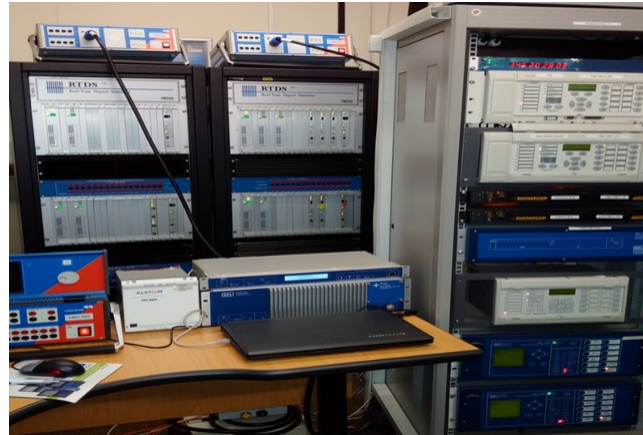
The RTDS Simulator installed at CPUT
