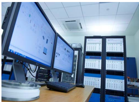
Figure 1: RTDS Simulator Installation
