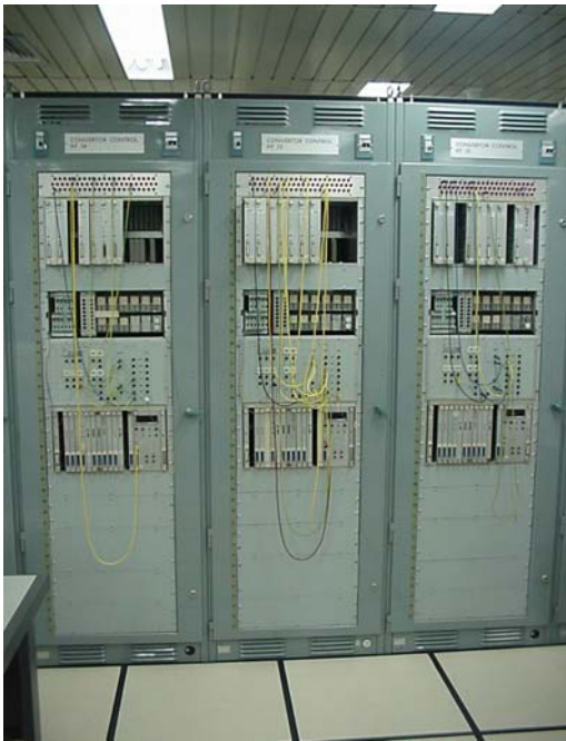
Fig. 1 - FURNAS HVDC control and Protection cubicles
