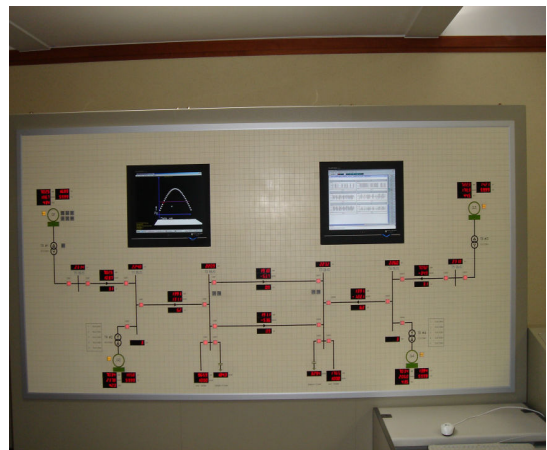
Fig. 4 A complete view of transmission mimic board
