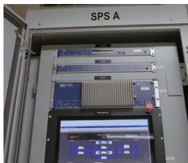
One of eleven Special Protection System cubicles assembled by SEL
