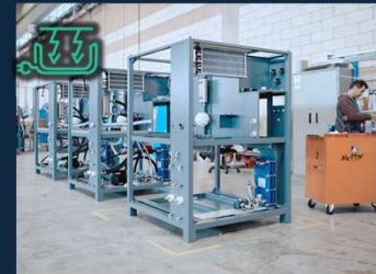
50 kW LH 2 Energy Plant
