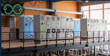
1 MVA PHIL Testing Hall
