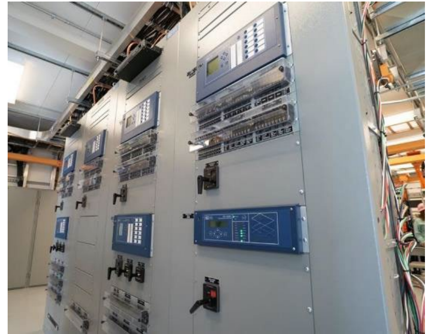
T400L relays installed in the substation [4]
