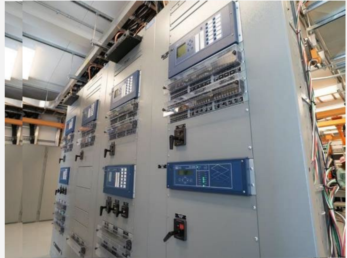
T400L relays installed in the substation
