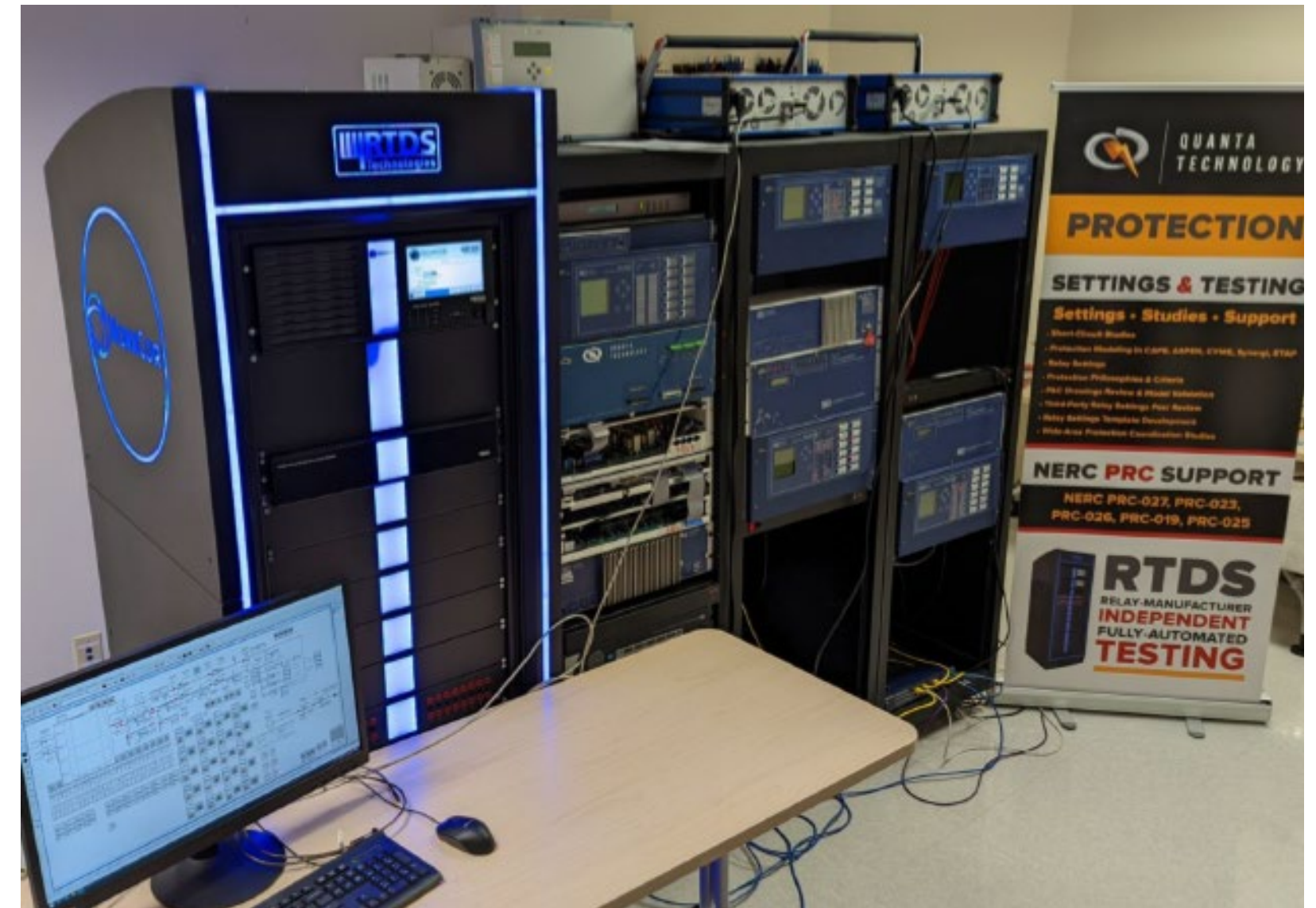
Quanta Technology's testbed for studying impacts of DER on protection for a utility customer
