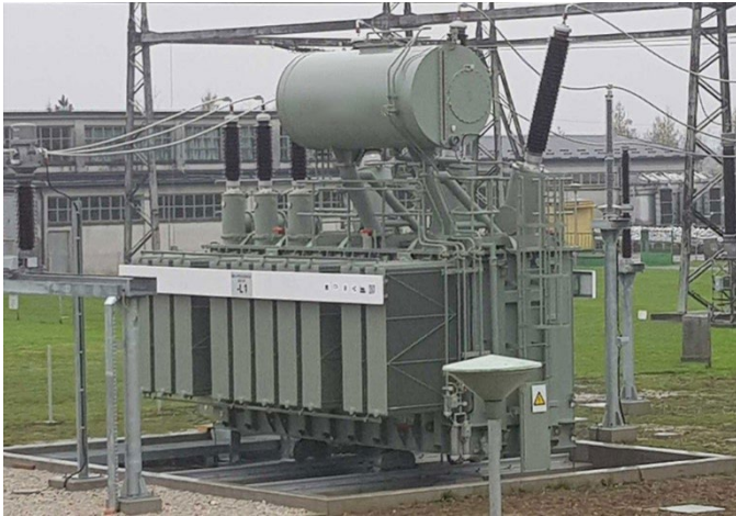
Fig. 3. An oil-immersed iron-core shunt reactor.
